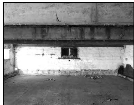
44. Gosford Road, Beccles, Suffolk. Wedge wire drying floor. [BB95/01927]
