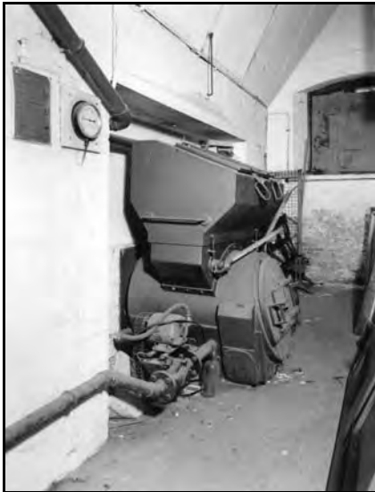
45. Suxé Furnace - Malthouse No 4 Weymouth, Dorset. [BB95/08083]
